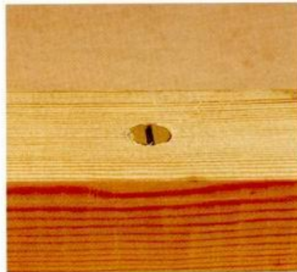
ABOVE: If all is well, the top face of the screw will be a clean fit, but fractionally lower than the surface of the wood.
