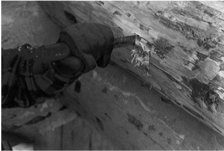
STEP 5: The rectangular hole may now be chiselled to accommodate the box.
