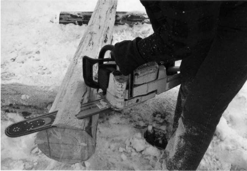
STEP 15: Correct procedure will guide the builder to the end of the log and very little touch-up work will be required.
