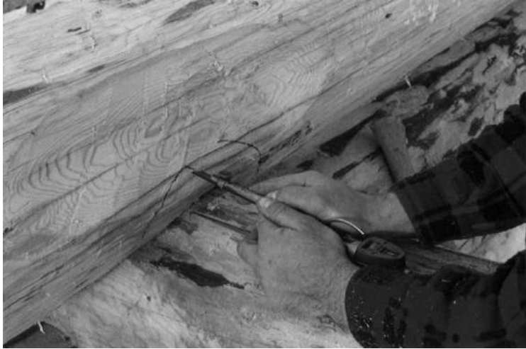
STEP 8: Scribe the notch, always keeping the dual level bubbles PERFECTLY LEVEL.
