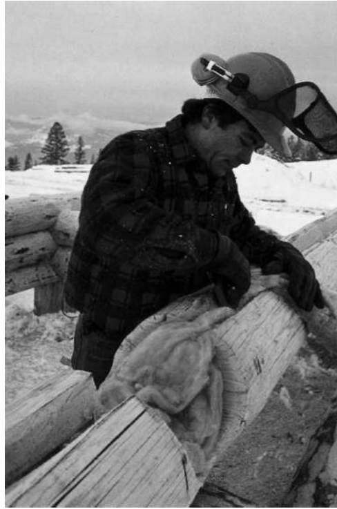
STEP 27: Once the log has been correctly fitted, insulation is stapled in the notch and along the lateral groove. (At the time of this publication, materials other than fibreglass are being experimented with and the reader may wish to choose an alternate insulating material).
